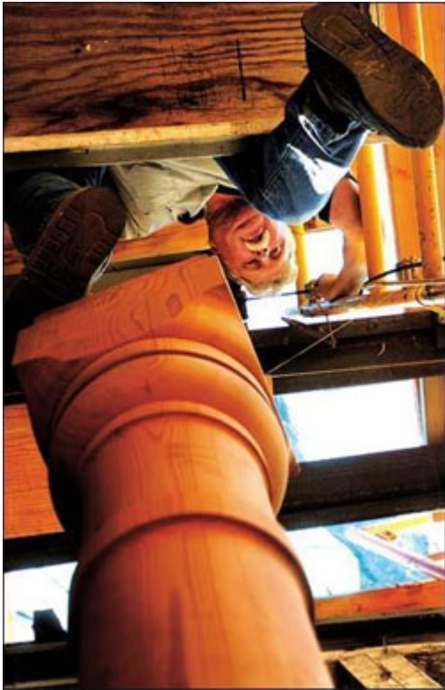
Mike Bordenkircher of the Hudspeth Corporation helps set a new column in place Thursday on the Bok Kai Temple in Marysville.
